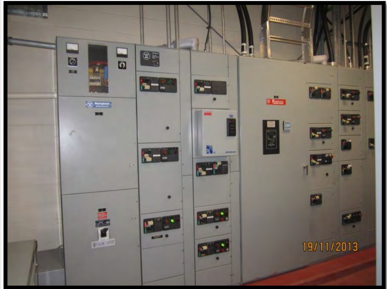
Motor Control Centre (MCC)
