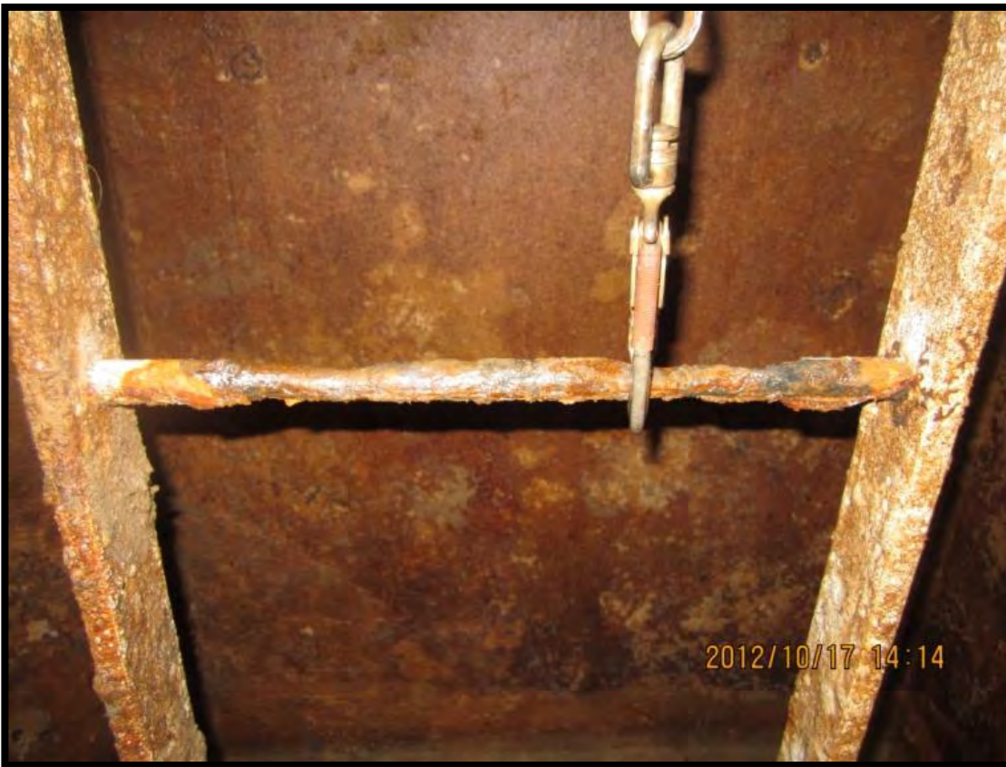
Photo 2 – Ladder Run Corrosion
