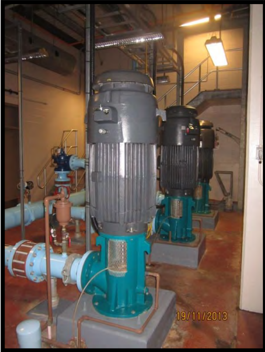
200 hp Distribution Pumps
