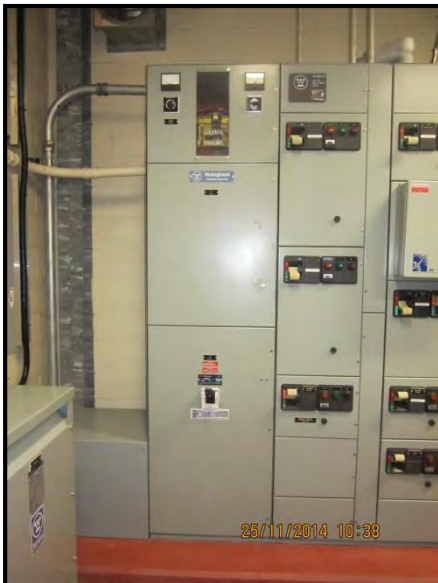
Main Incoming Breaker
