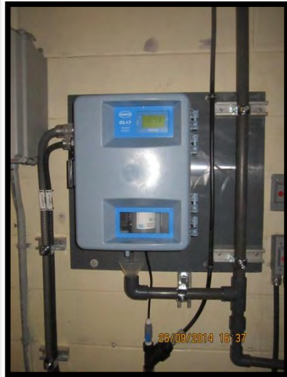
Hach Analyzer installed in 2014
