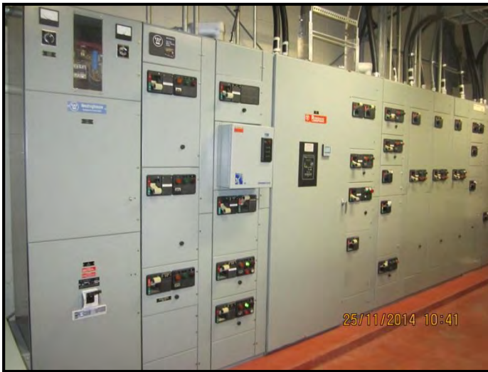
Motor Control Centre
