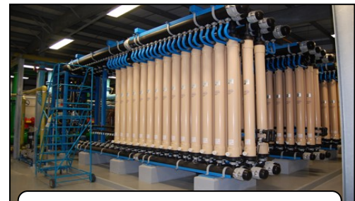
Filtration / Treatment systems in
