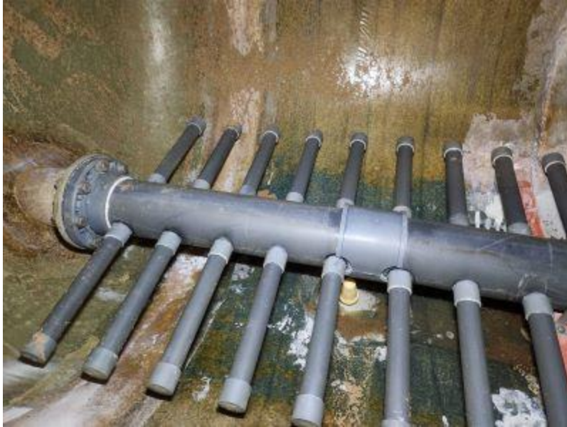
Inside the filter tank once all the sand and gravel are removed.
