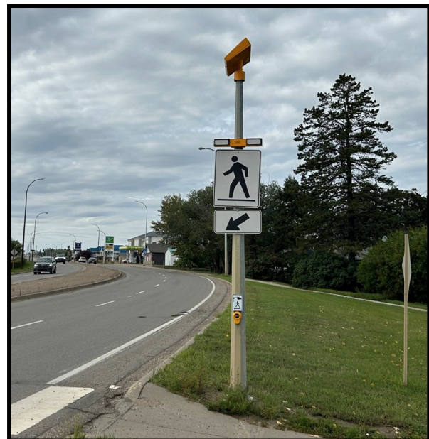
New Pedestrian Crossing Lights
